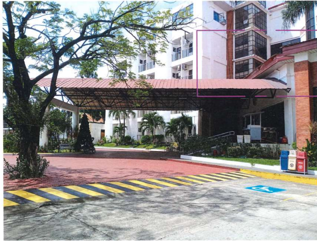
EXISTING CONDITION OF FASCIA FLASHING
